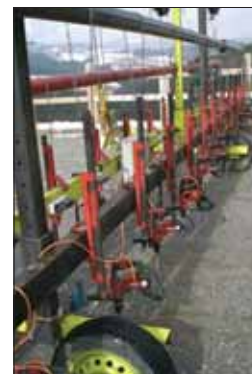
◆◆◆ Holes for interface shear reinforcement bars can be drilled quickly using Hilti's specially developed special multi-point drill wagons
