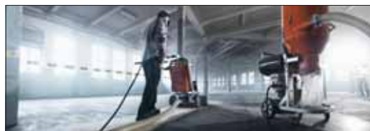
♦♦♦ Floor grinding and polishing of concrete has shown considerable growth in recent years
