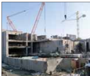
◆◆◆ 28,000 m of diamond wire was used to cut the concrete into blocks as large as 100 tonnes
